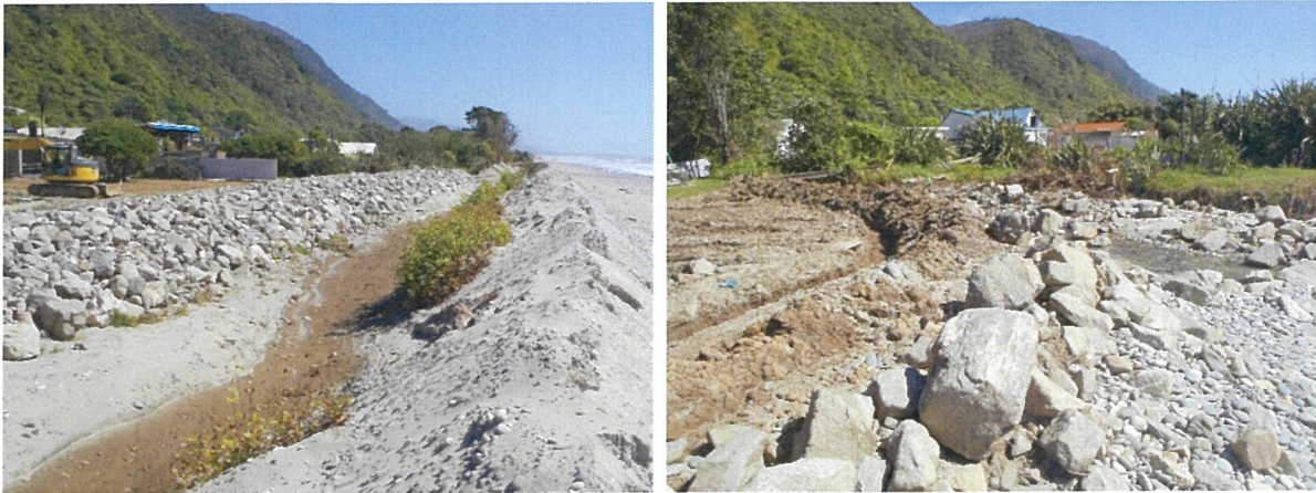
Figure 4 Recent hard defences under construction north of Bradley Stream (G4) where the drain diversion bund failed. Left, 158-160 Torea St; Right, 154 Torea St. [Source: M Allis 22-11-2016].
